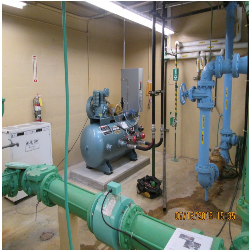
Hydroburst tank inside Pumphouse Building
