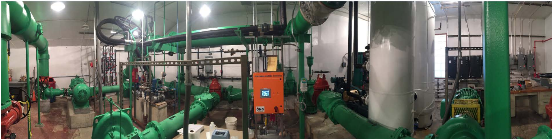
Panoramic of inside pump station
